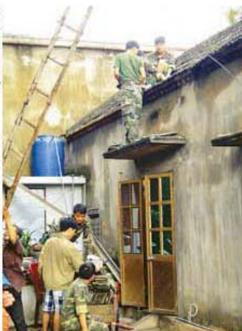
Soldiers help residents to repair their homes after the storm attacked An Lu commune in Hai Phong. (Photo:SGGP)
